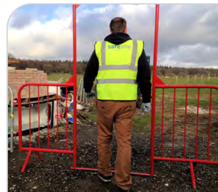
Pedestrian walk through barrier
